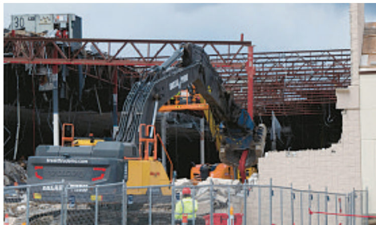
Demolition crews are taking down the former Round Lake Beach Kmart, with the site to become a new Target. The building has sat vacant for years. JOE STATES/PIONEER PRESS
