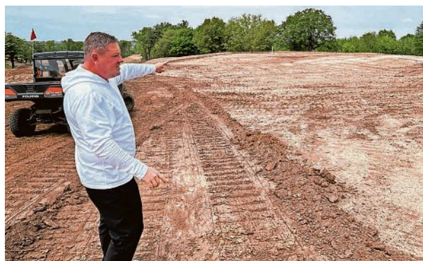
Finkbine Golf Course General Manager Josh Clay explains the design of holes 10 and 11 at the reimagined course, now under construction in Iowa City. PROVIDED BY ERIN JORDAN/IOWA CAPITAL DISPATCH
