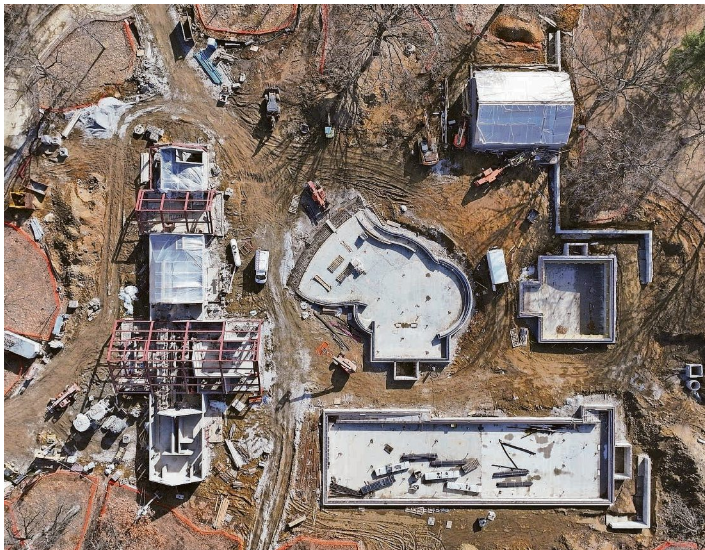
An aerial view shows the ongoing construction of City Park Pool. The pool was slated to open during Memorial Day weekend, but has been pushed back to a midsummer opening. PROVIDED BY THE CITY OF IOWA CITY GOVERNMENT
