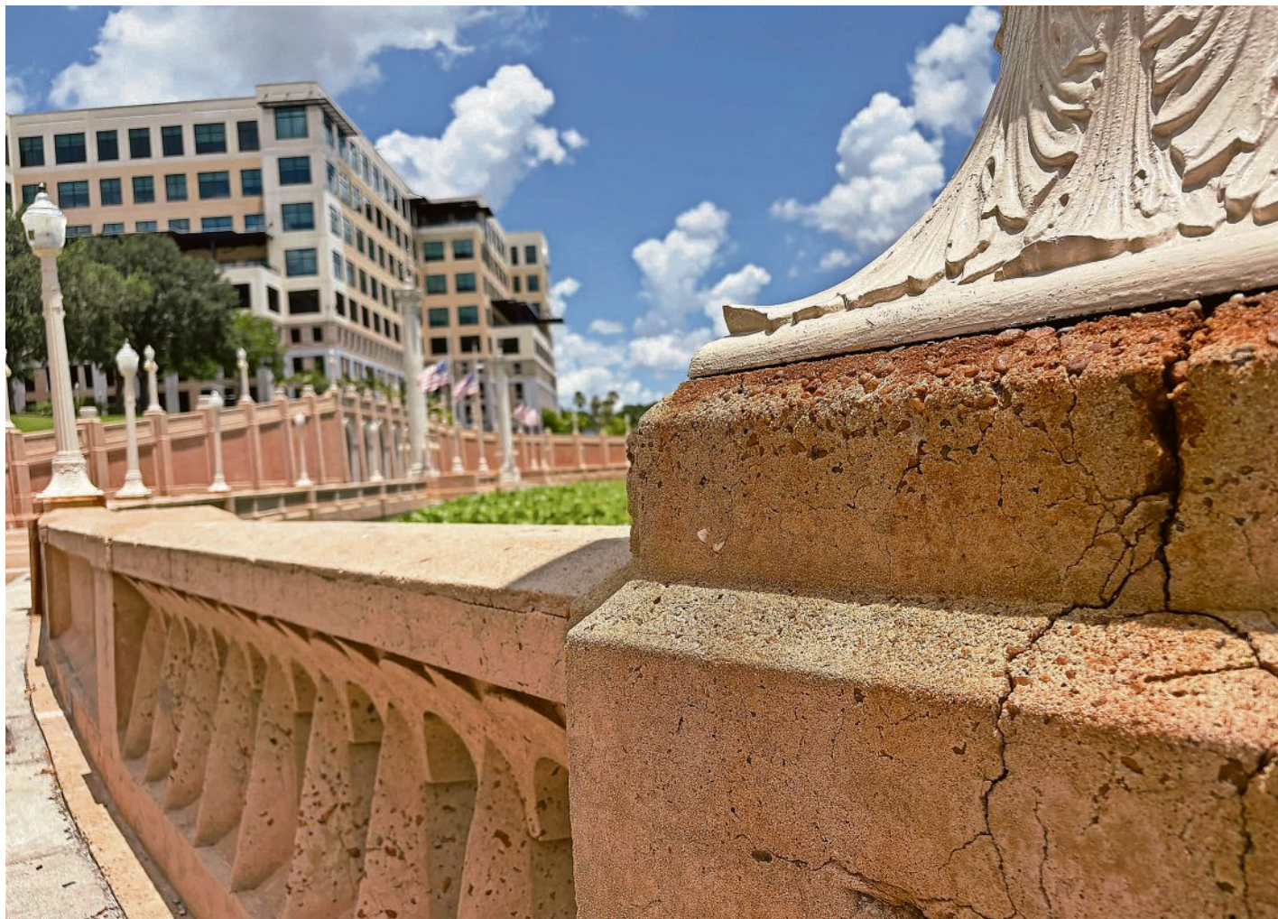
Lakeland's iconic France Langford Promenade and The Loggia are cracking, showing signs of damage and ongoing water instruction ANDY KUPPERS/THE LEDGER
