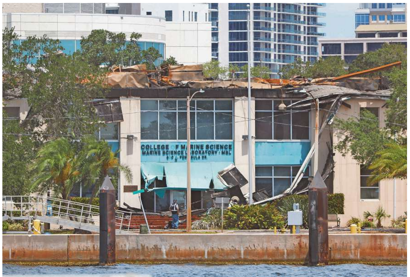
Questions about the condition of the roof of the Marine Science Lab on the University of South Florida St. Petersburg campus have been raised after the fire on Saturday. (JEFFEREE WOO | Times)
