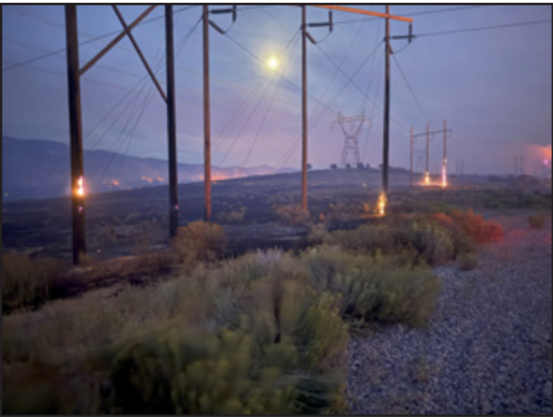
Poles supporting Tri-State Generation and Transmission Association power lines burn during a wildfire in Rio Blanco County this summer.
