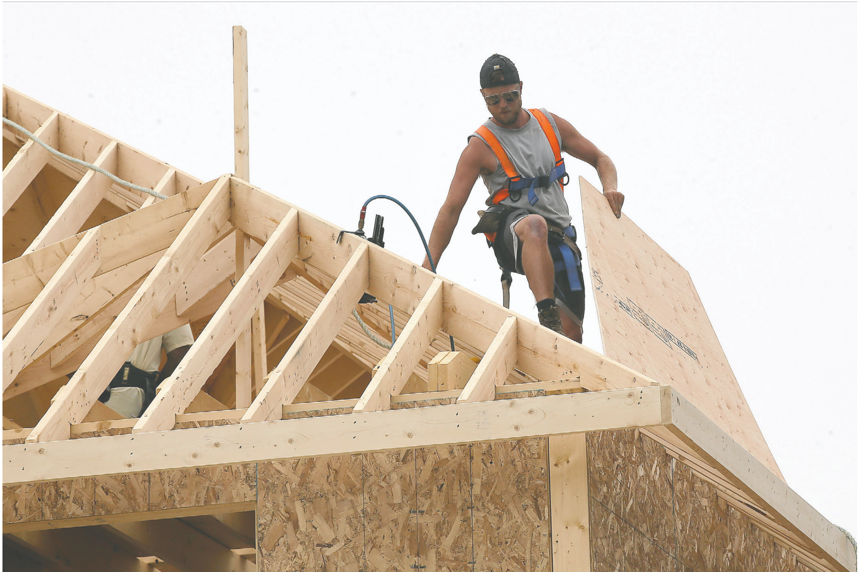
The provincial and federal governments have set aside $8.8 billion to cover housing-related infrastructure costs in an effort to spur development. DAN JANISSE
