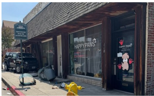
A car crashed into a three-unit building in Monrovia on June 21, leaving three businesses unable to conduct business while awaiting repairs. COURTESY OF MICHAEL DELGADO
