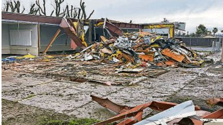
Planada Elementary School, built in 1955 below flood level, damaged by heavy rains and a levee break on Jan. 6, 2023. PROVIDED BY PLANADA ELEMENTARY SCHOOL DISTRICT
