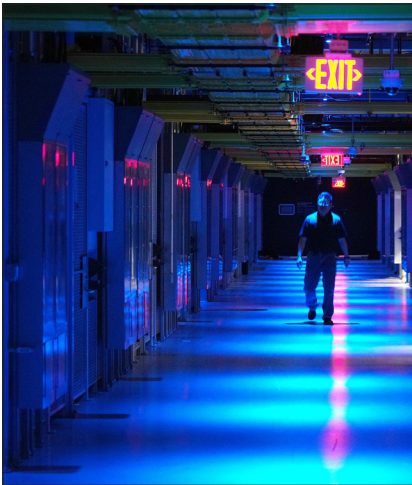
Artificial intelligence relies on data centers, like this one in San Jose, which are having a profound impact on demands for energy and water in California and around the world. JIM WILSON THE NEW YORK TIMES
