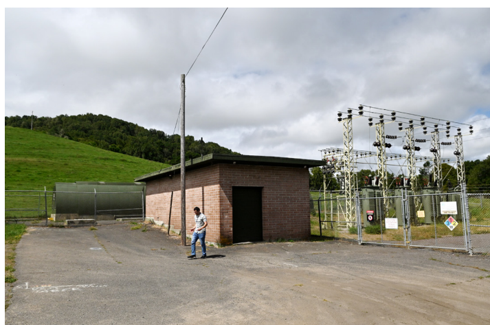
The 65-year-old Tocaloma pump station in rural Marin is getting a $12.1 million makeover.
