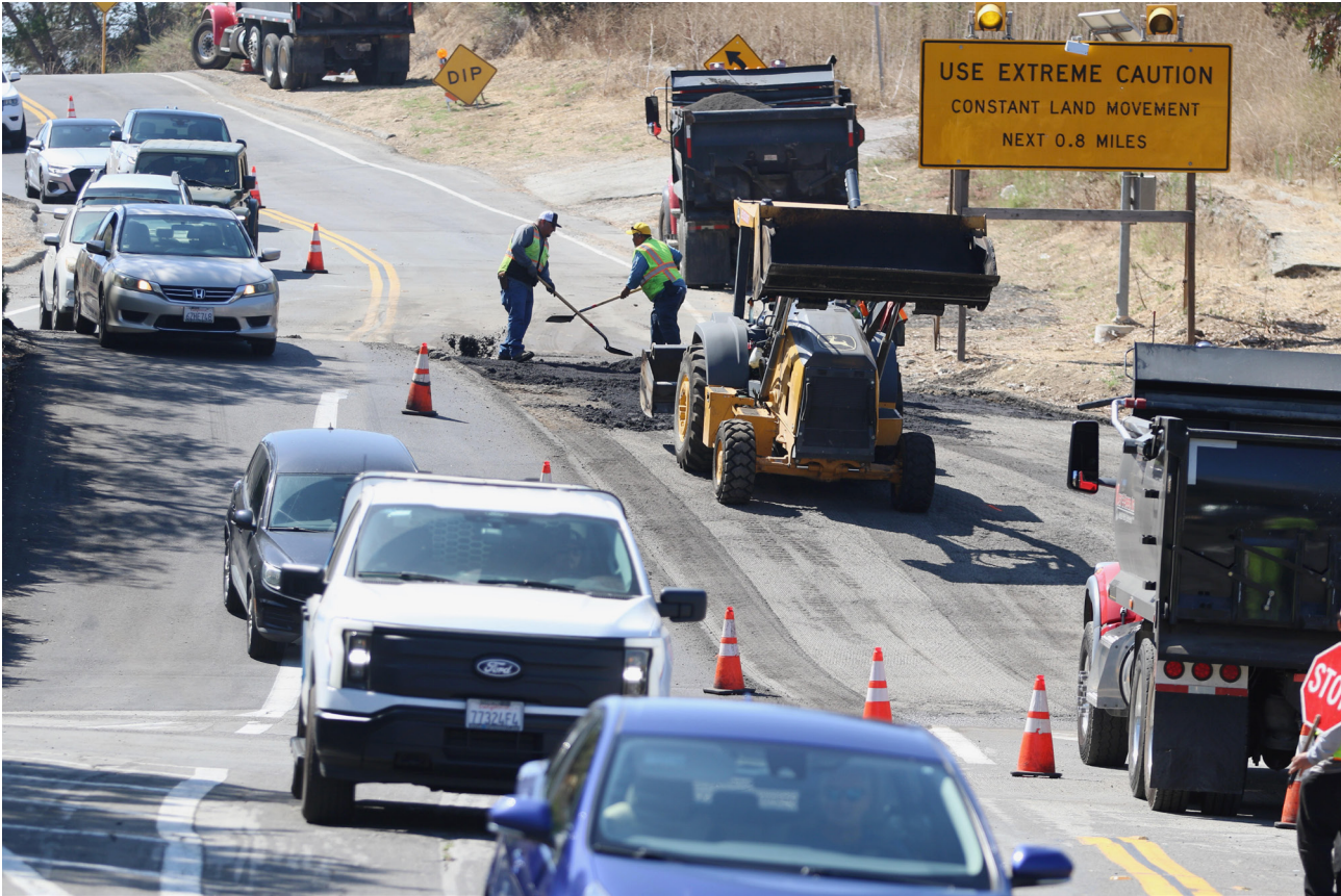
Traffic is temporarily reduced to one lane for roadway repairs on June 15 along a portion of Rancho Palos Verdes Drive South, especially prone to landslides in Rancho Palos Verdes. PHOTOS BY HOWARD FRESHMAN
