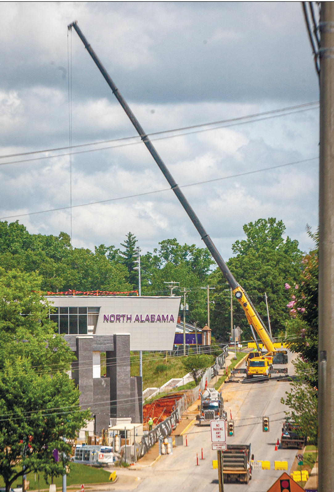
A crane boom extends over Pine Street near the University of North Alabama as crews work Thursday to install speakers on the video scoreboard at the new Bank Independent Stadium in Florence. [PHOTOS BY DAN BUSEY/TIMESDAILY]
