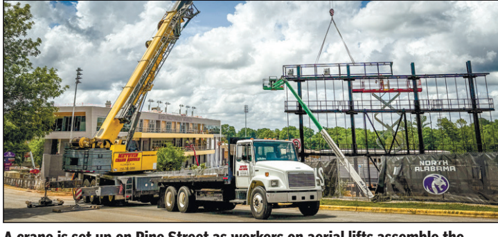
A crane is set up on Pine Street as workers on aerial lifts assemble the video scoreboard structure at the new Bank Independent Stadium on the University of North Alabama campus Thursday in Florence. Pine Street was closed to allow the crane to hoist speaker equipment for the scoreboard.
