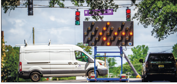
A detour arrow board directs traffic at the intersection of Irvine Avenue and North Pine Street near the University of North Alabama campus as Pine Street is closed Thursday in Florence to allow crews to install speakers on the video scoreboard at the new Bank Independent Stadium.
